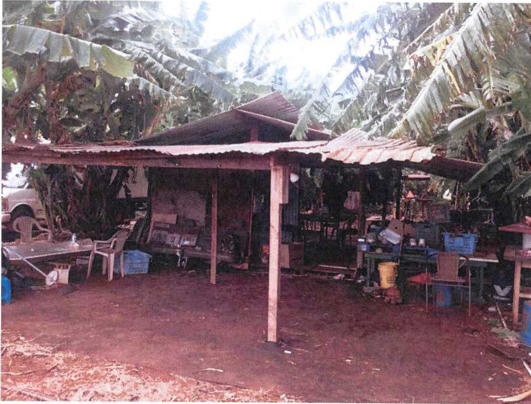
Unpermitted structure on the License area
