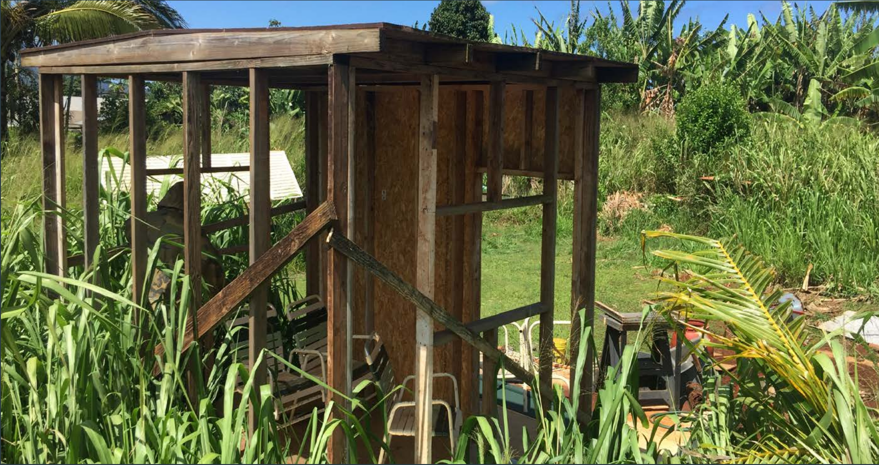
Unpermitted structure located on State property.
